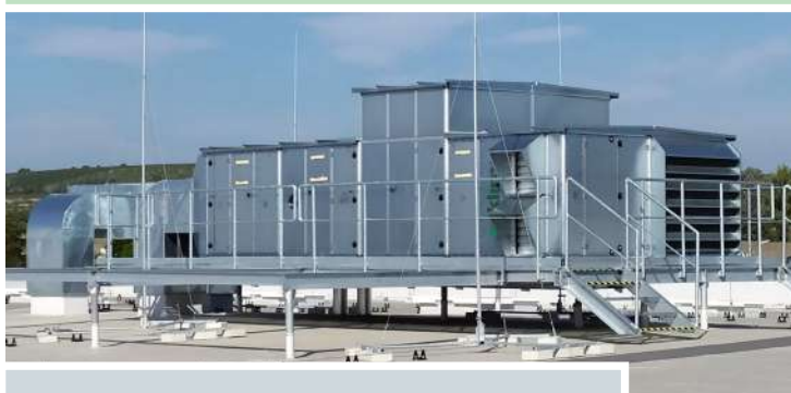
Air handling units
